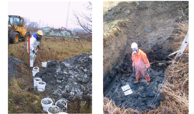
Collecting sample of polluted soil to contractors. Half masks were needed because of the odour.
